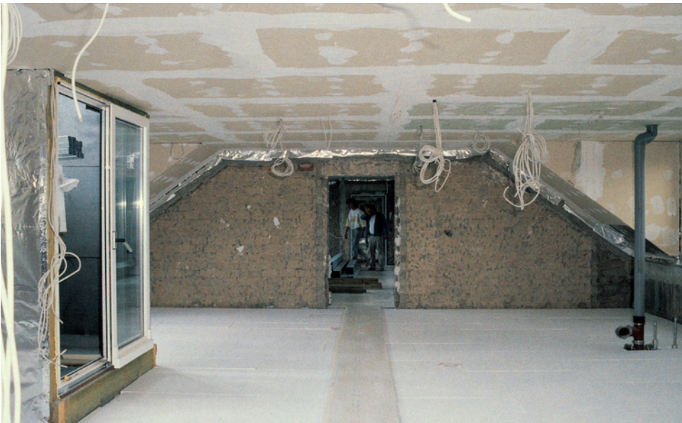
Attics in existing apartment buildings, like this one in Aschaffenburg, Germany, were converted into two-bedroom apartments.
