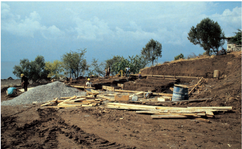
Europe Division construction sites in Turkey included Sinop on the Black Sea.
