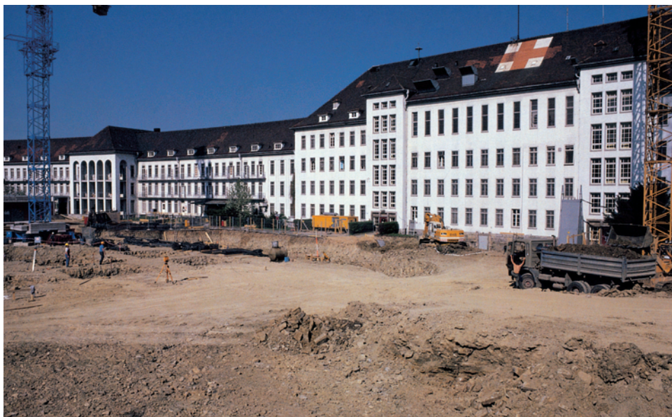
Construction began in March 1987 on the addition to the Army hospital in Würzburg, Germany.
