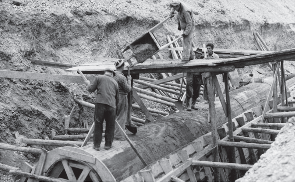
Building Camp Roeder involved installing and constructing all utilities, including a sewer system.
