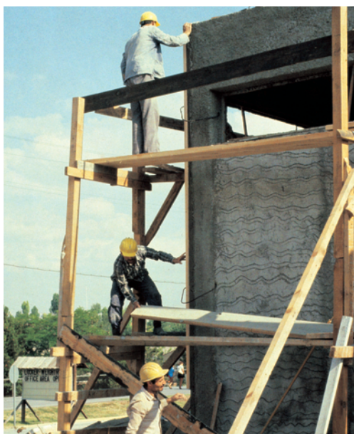
Construction of even this simple warehouse near Ankara involved special measures to strengthen the Turkish construction industry.
