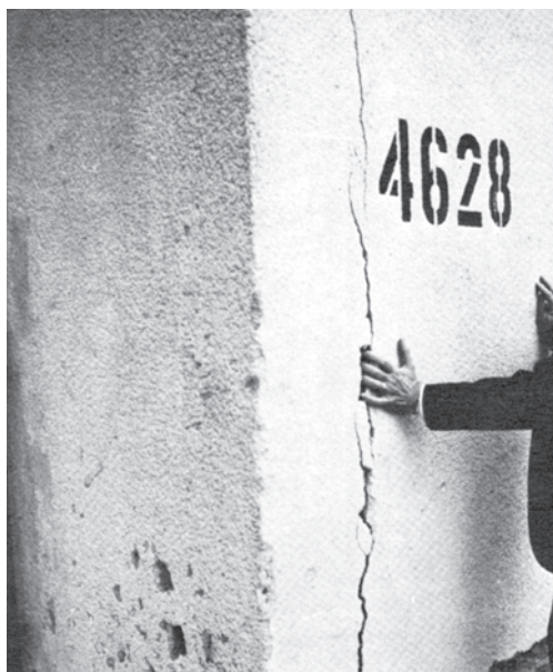
Housing suffered from a backlog of delayed repairs. This family housing unit in Giessen, Germany, shows signs of severe structural cracking.
