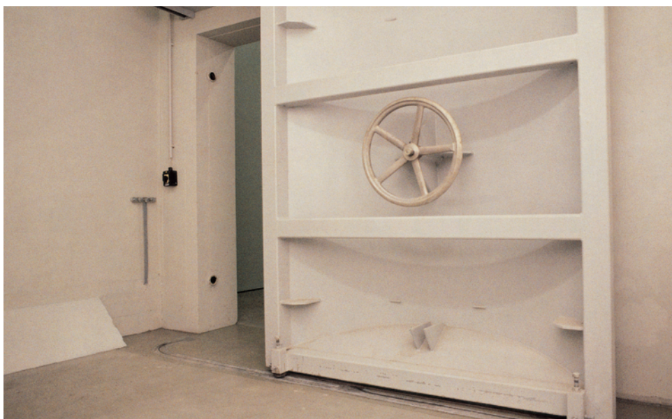
To protect ammunition at LRSP sites, the Europe Division fitted bunkers with heavy doors, like these in Miesau, Germany.
