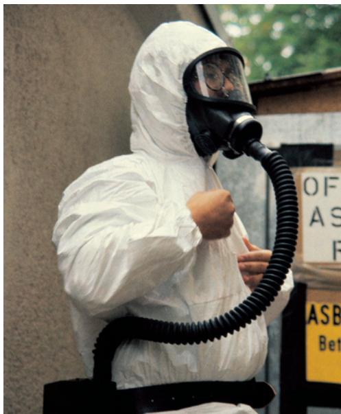
Contractors wore special protective suits while removing asbestos from school buildings in Europe.
