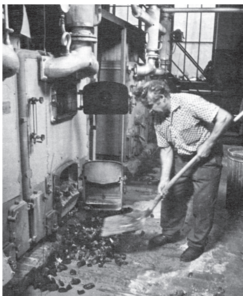
Coal-fired boilers, like this one at Warner Barracks in Bamberg, were prevalent in the 1960s and 1970s.
