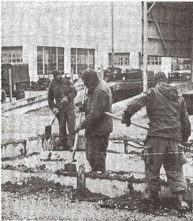
PRE-FAB SHELTER-A Foundation is being poured for a prefabricated shelter on Custer Hill during FTX. The 15' by 24' shelter will be used for storage. Facing the camera is PFC William Delgado.
