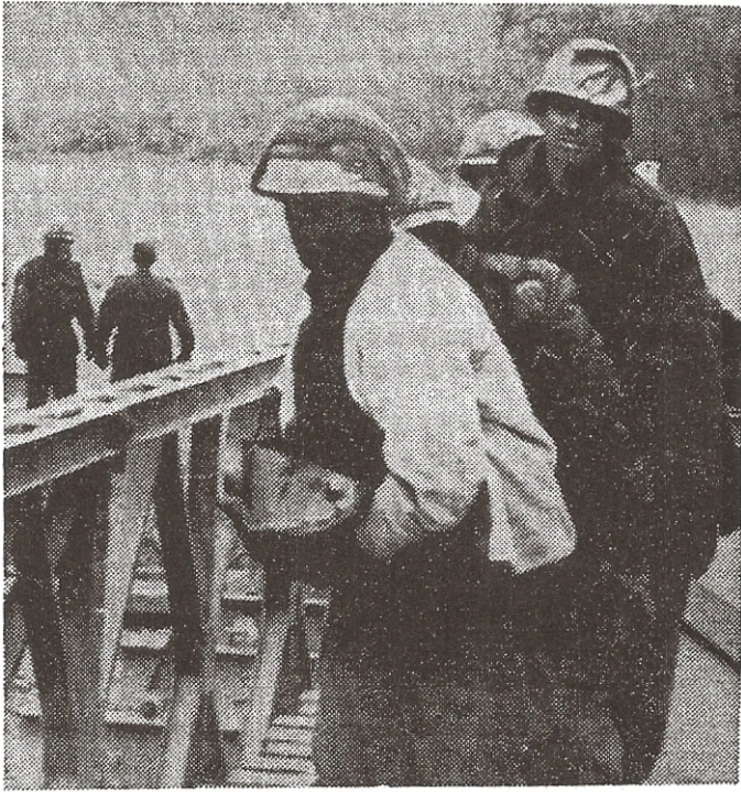
BEAM FOR FTX-SP4 Earnest Hurt, PVT Terry Lee, and SP4 Charles Tacket carry a beam for the heavy-duty prefabricated bridge.
